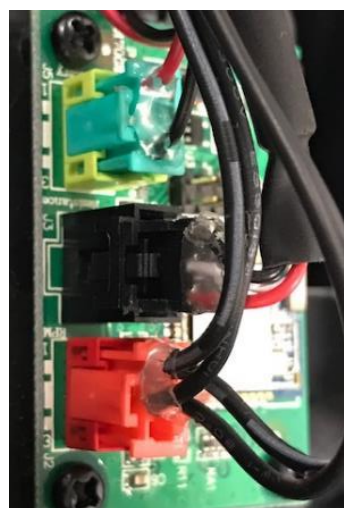
Figure 5 - Wires Connected to LCB
