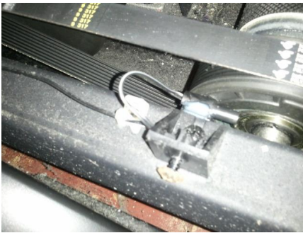
Incorrectly Mounted Sensor
