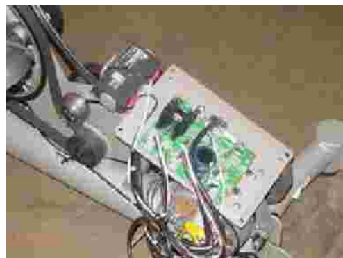
Figure 14b - Power board cables disconnected (R916 shown)
