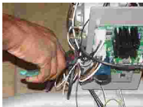
Figure 17 - Cut cable tie
