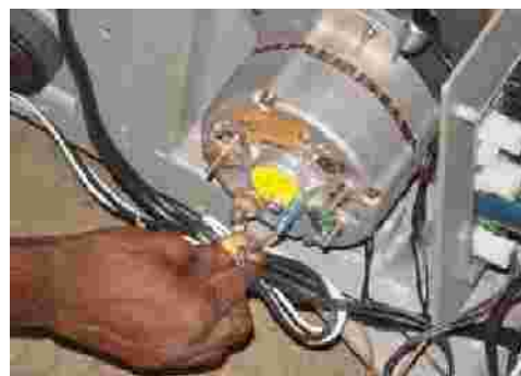
Figure 23 - Detach all cables from alternator
