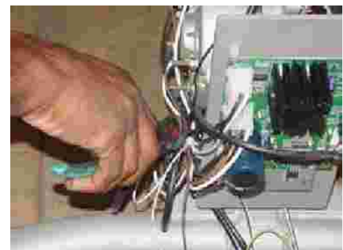
Figure 20 - Cut cable tie
