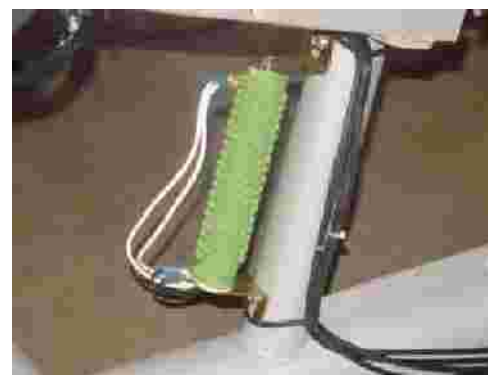
Figure 9b - Resistor wires (R916)
